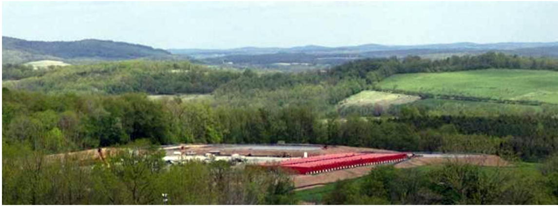
Photo 6.3 - A representative view of a newly constructed water impoundment area (New August 2011)
