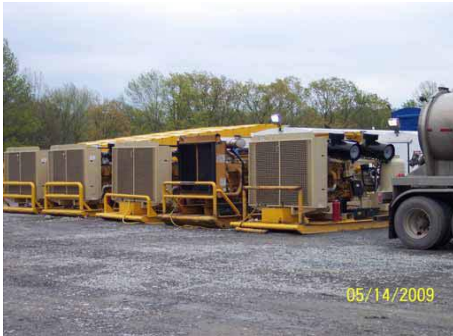
Photo 6.6 - Electric Generators, Active Drilling Site (New August 2011)
