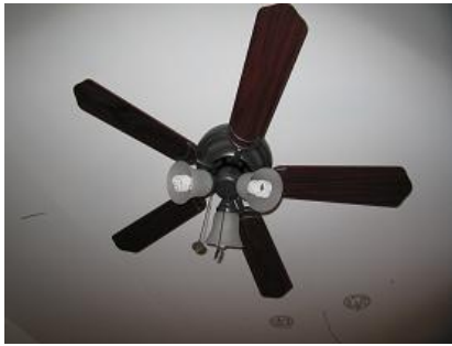
Ceiling fan and light
