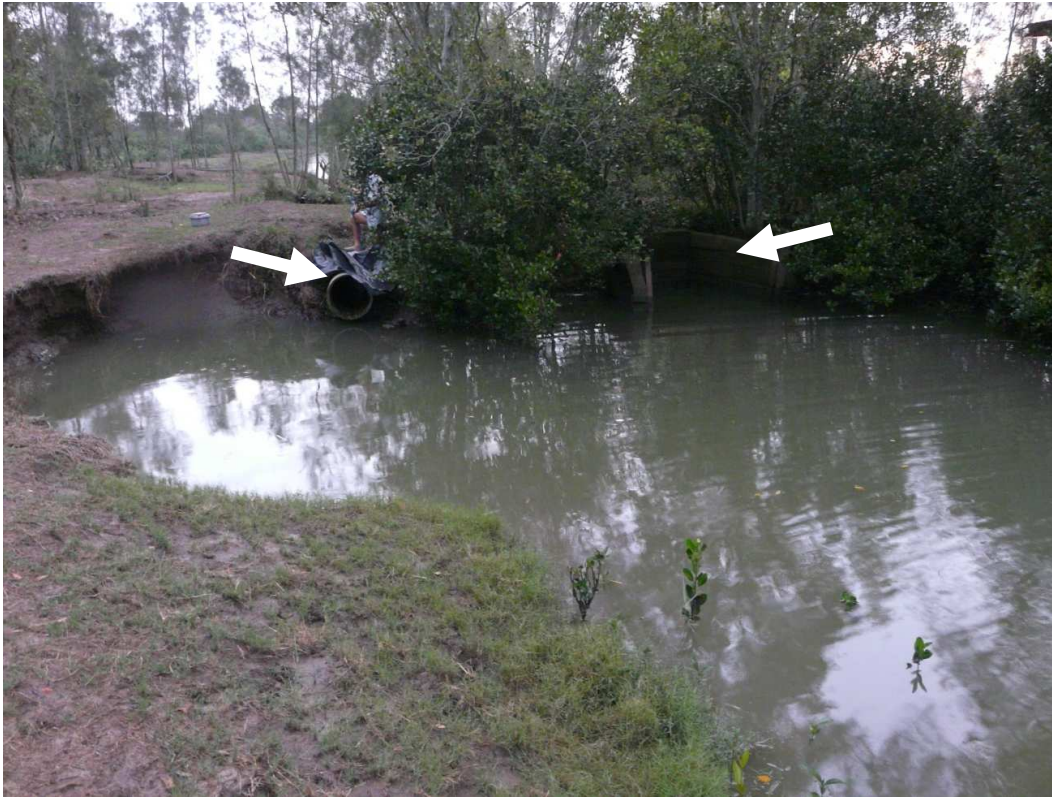
Figure 2. Location where intake of IP1 is blocked by dual floodgates (right arrow), while the overflow pipe is evident to the left (left arrow). The intake was blocked on 2 nd December.
