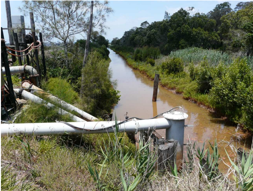
Figure 5. Northern end of western effluent channel at farm 3, looking south. The canal was blocked here at the northern end around 11 am on Monday 5 th and is beginning to fill up at quite a rate. This will need to be decontaminated before being allowed to empty again into the river.
