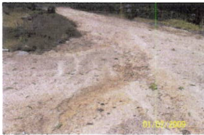
Damaged driveway B. Kilner
