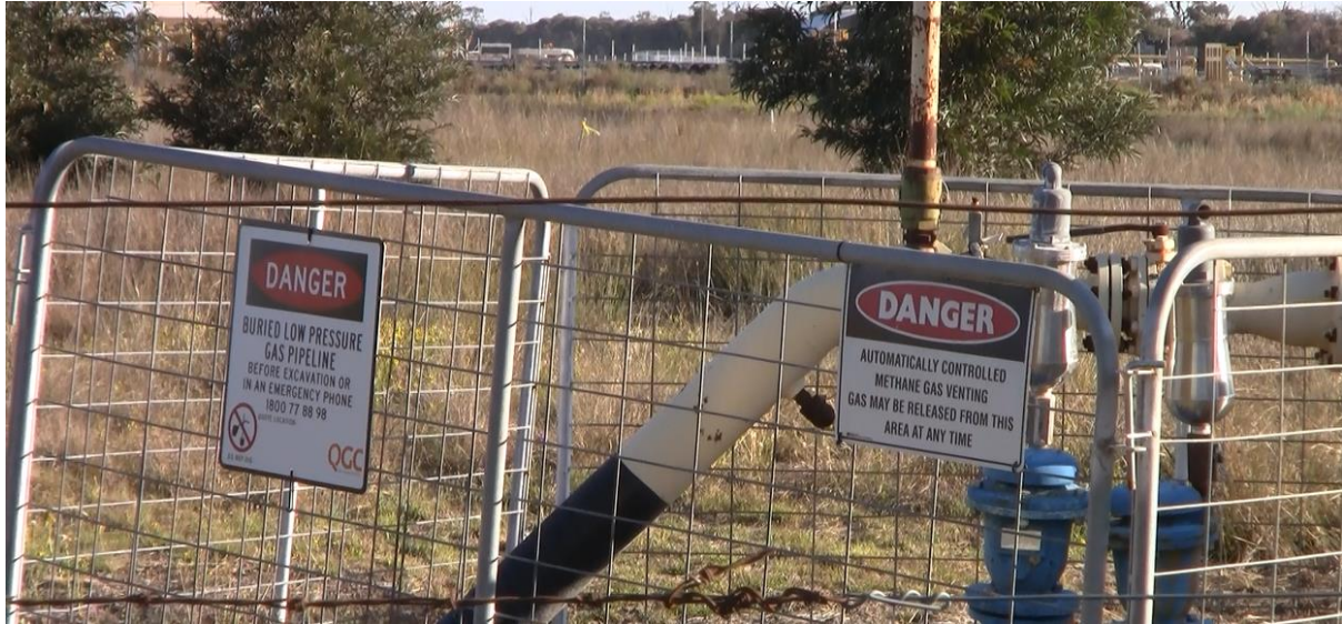
METHANE VENTING SIGN, KENYA GASFIELD, TARA REGION PHOTO COURTESY OF LOCAL RESIDENT
