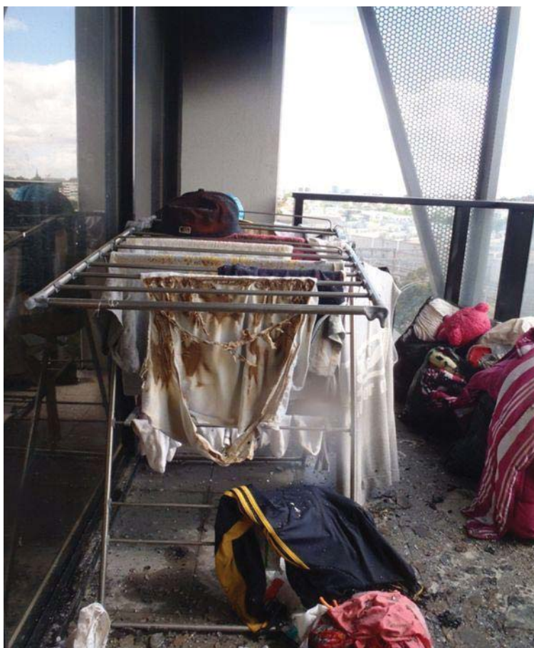
Figure 11 - Combustibles stored on one of the balconies.
