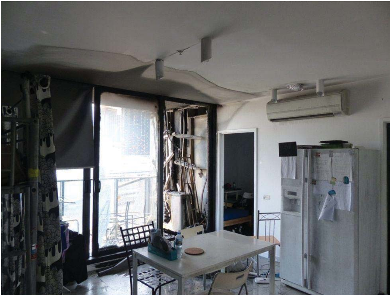
Figure 5 – Picture 4: Inside kitchen looking towards double glass sliding doors leading to balcony area & bedroom 2.
