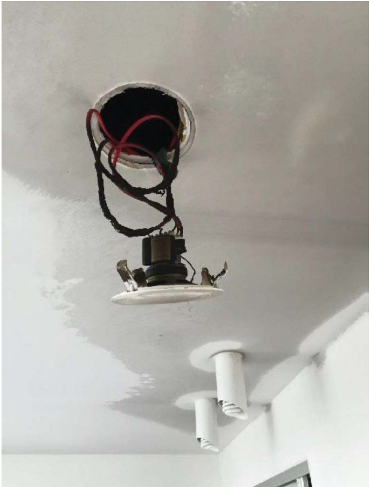
Figure 20 - EWIS Speaker and wiring
