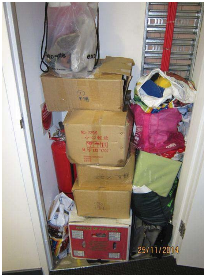
Figure 13 - Fire extinguisher cupboard on Level 6.
