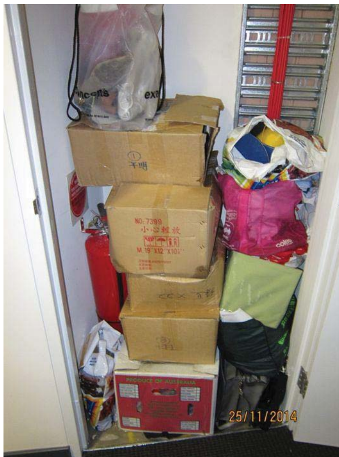
Figure 13 - Fire extinguisher cupboard on Level 6.
