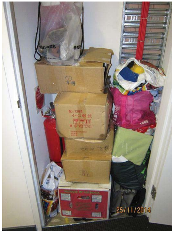
Figure 13 - Fire extinguisher cupboard on Level 6.
