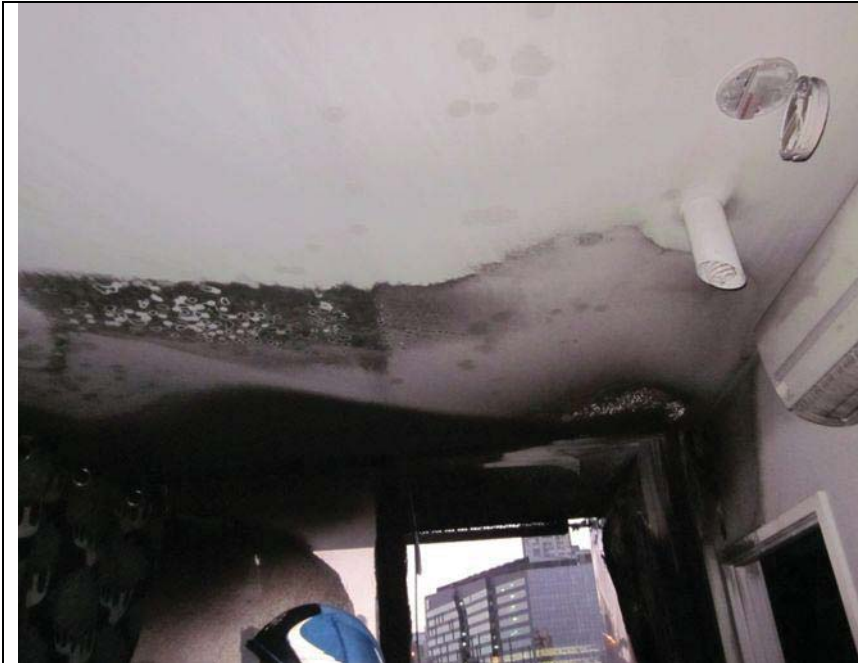
View of damaged wall and smoke detectors made inoperable. Others were covered over.
