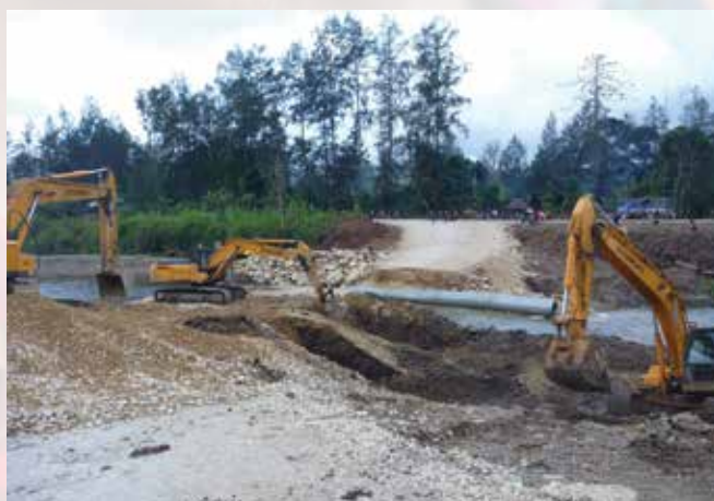
Work underway on the road outside Tari 2011. Photo credit: James McIlraith/ University of Otago.
